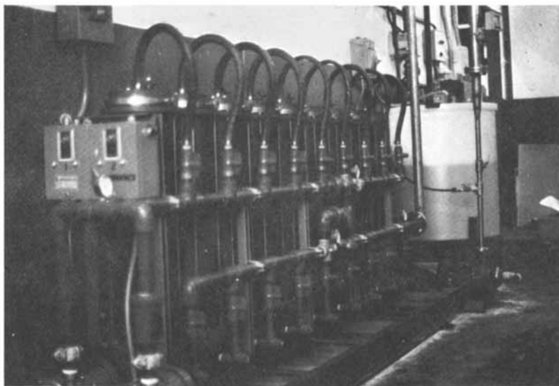
Figure 9. A bag filter system used for pretreatment prior to an oily waste application. We are using 5- \mu -rated bags which we feel are approximately equal to 15- \mu cartridge filters. Bags are valuable because the waste that is collected can be thrown away.
